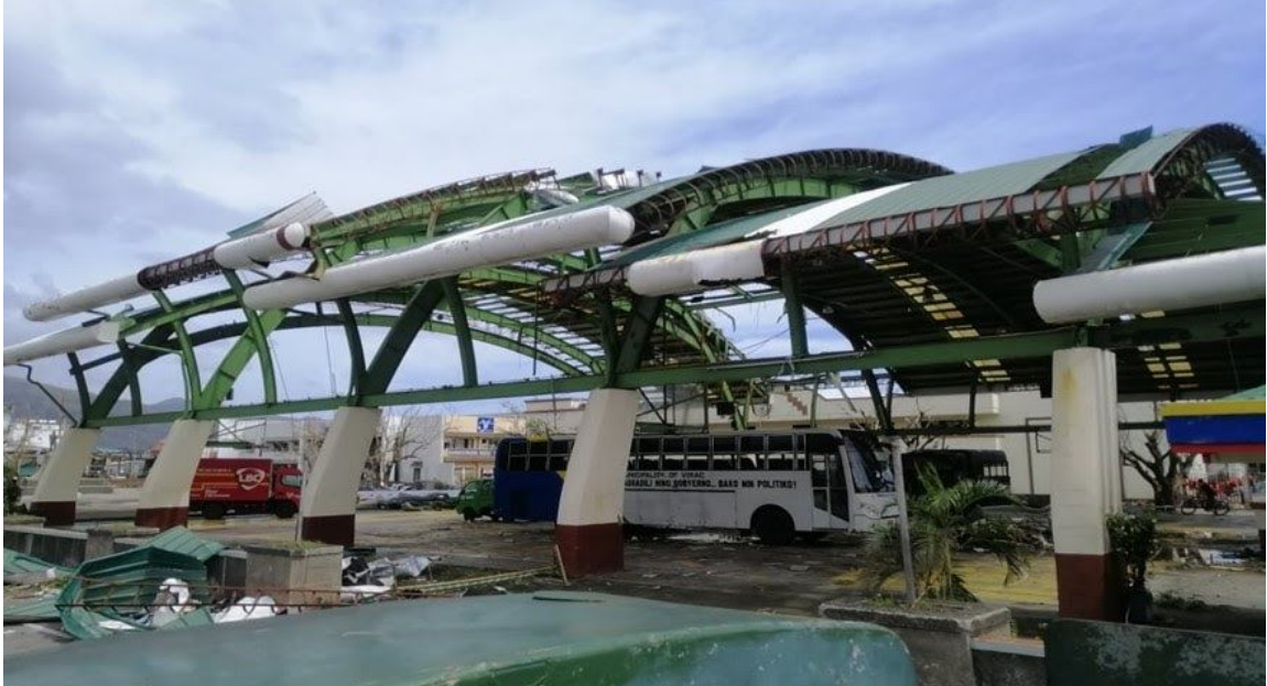
Figure 4. Wind damage to infrastructure in Catanduanes province (Bicol Region) (Source: OCD )
